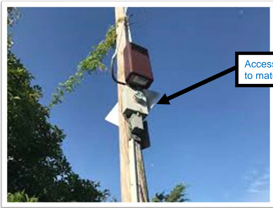
Figure 5.1 - Unacceptable Installations on Utility Poles
