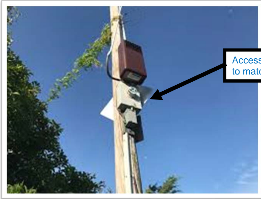
Figure 5.1 - Unacceptable Installations on Utility Poles
